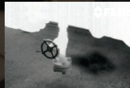
METHANE LEAK AT NATURAL GAS FACILITY SITE
