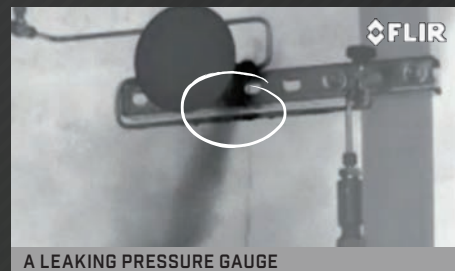
A LEAKING PRESSURE GAUGE
