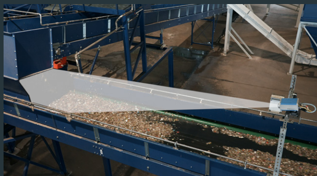
PYROsmart® one always keeps belt transfer points in view and detects critical temperatures in free-falling material.
